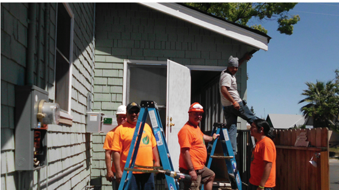
Left: Five of the volunteer workers take a moment to smile for the camera before getting back onto the roof for installation.
